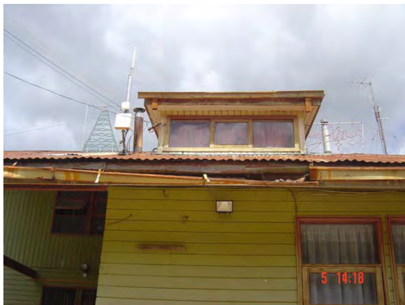
Fig 1: Corrosion to roof cladding and gutter collapse following 200 mm of ashfall in Futaleufu, Chile following the 2008 Chaiten eruption (Photo: T. Wilson).
