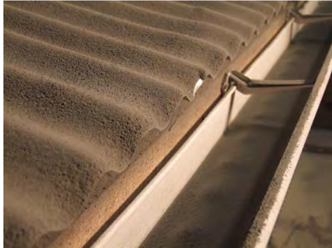
Fig. 10. Deposition of ash on roof with 15^\circ angle. The roof surface was mantled with ash, with some infilling the spouting at end of testing (Photo; S. Hampton).
