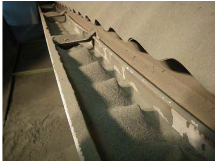
Fig. 11: Deposition of ash on a roof tilted at 25^\circ . There is asymmetric ash accumulation in guttering, with piles accumulating beneath troughs. Ash distribution is grain size controlled, with coarse ash depositing on outer edge of spouting. Fine ash accumulates within the gutter until buoyancy caused the ash to bypass the spouting. In distance, ash accumulation is prominent on guttering bracket, limiting ash accumulation beneath.
