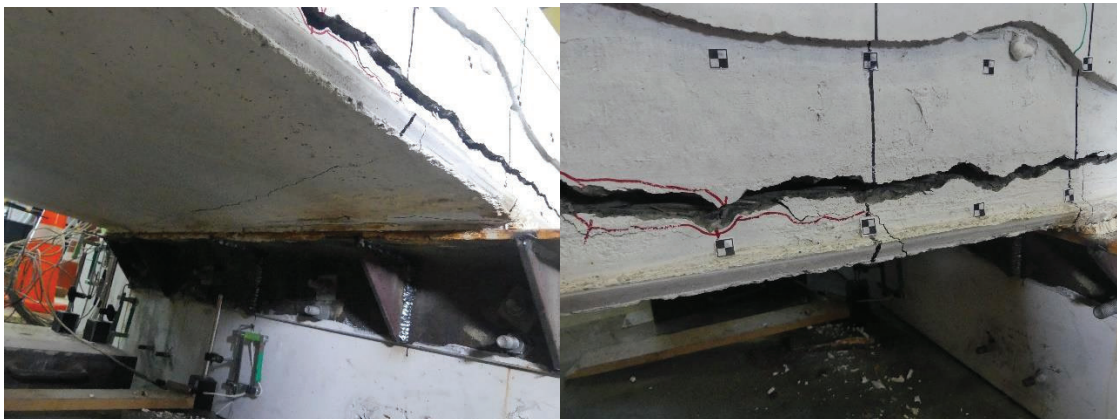
Figure 25: Extensive Soffit Cracking at +4.0% drift
