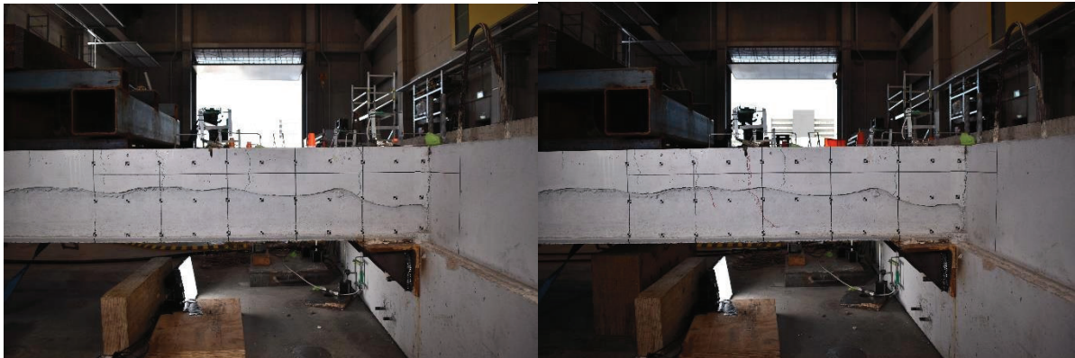
Figure 18: West Side of Specimen 4 Directly Prior (Left, -1.0% Drift) and After (Right, -1.6% Drift) NM Crack Initiation
