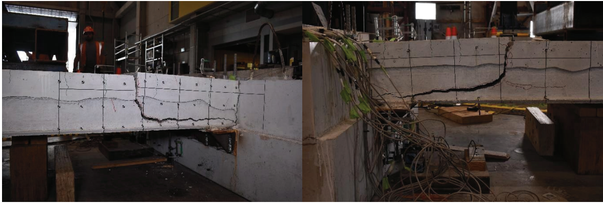
Figure 22: East Side of Specimen (Left) and West Side of Specimen (Right), the Residual Crack at 0% Drift
